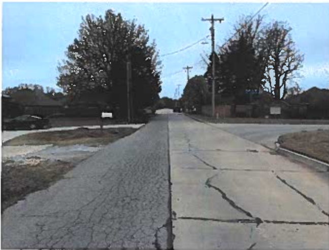
Looking south on Davidson Dr. Example of half street improvements on one side eventually being improved by another half street improvement further south.
