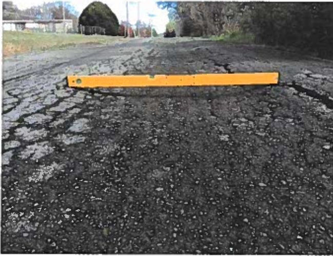
Looking north on Davidson Drive, east side of roadway. Note the presence of rutting and alligator cracking.
