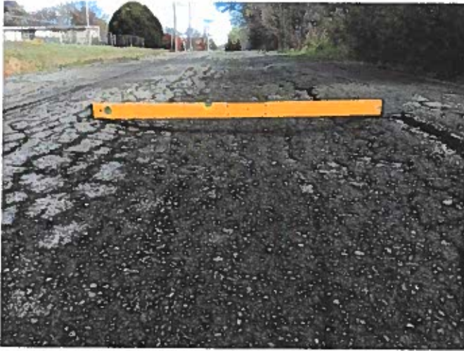
Looking north on Davidson Drive, east side of roadway. Note the presence of rutting and alligator cracking.
