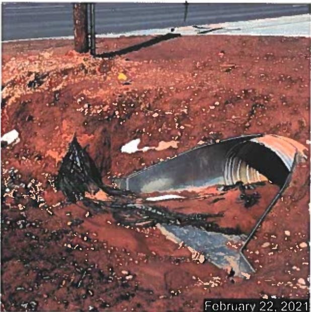
Upstream end of drainage culvert going under newly constructed driveway for Lot 1
