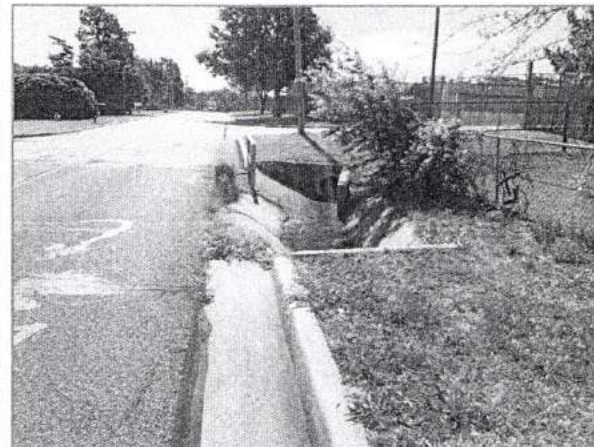
Looking east on E Main Street. Open paved ditch/ Inlet at Northeast corner.
