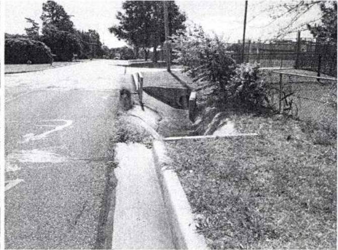
Looking east on E Main Street. Open paved ditch / inlet at Northeast corner.
