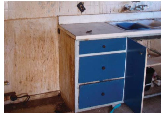
Example of deteriorating housing condition
