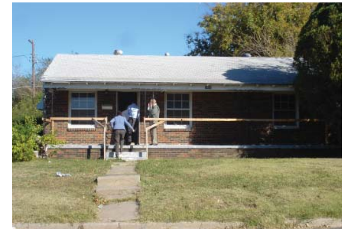
Example of deteriorating housing condition
