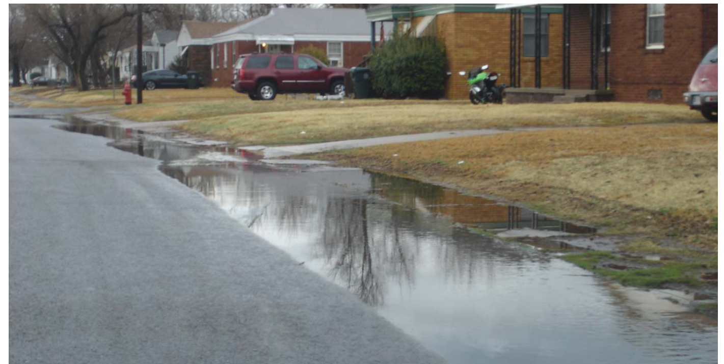
Storm water ponding during one inch rain
