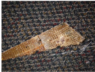
Photo #13 Mastic under carpet
