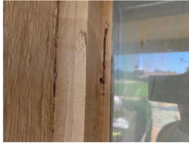
Photo #21 Outside window caulking
