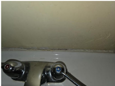
Photo #16 Sink caulking
