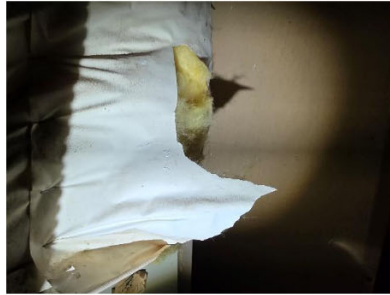
Photo #4 Duct insulation
