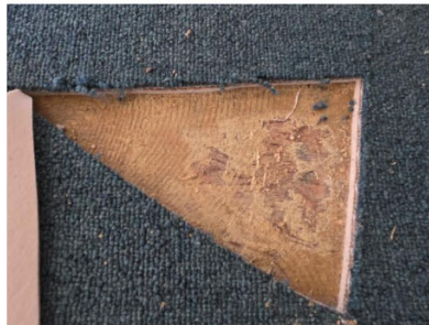
Photo #6 Blue carpet mastic
