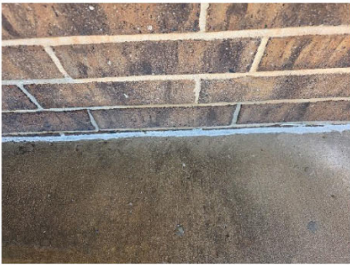
Photo #22 Outside wall caulking
