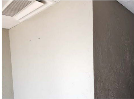
(I-01) Asbestos Detected
