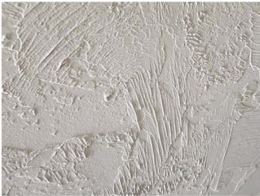
(I-02) Asbestos Detected
