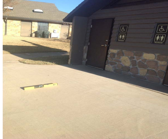
2. Comment: Violation AR_I1
