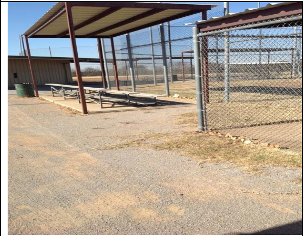
3. Comment: Violation AR_I2
