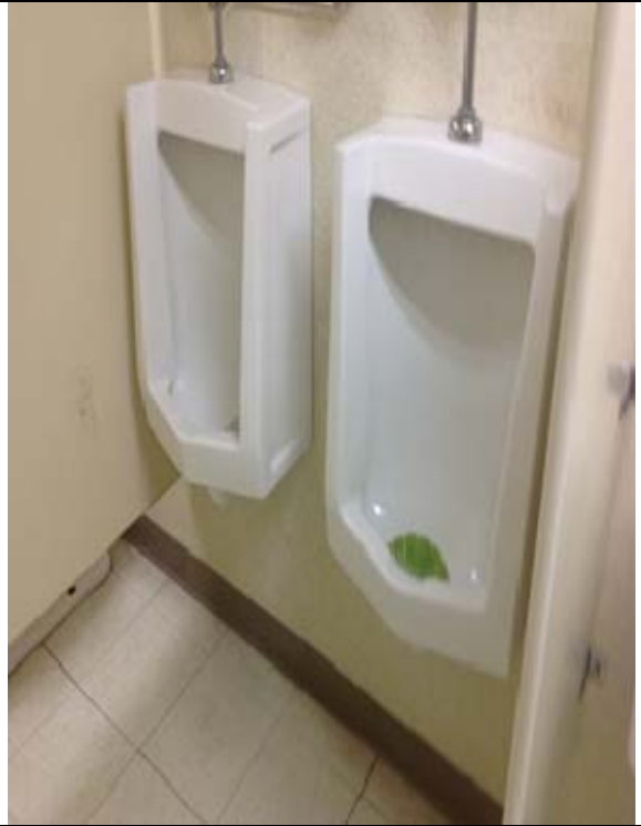
14. No accessible urinals
