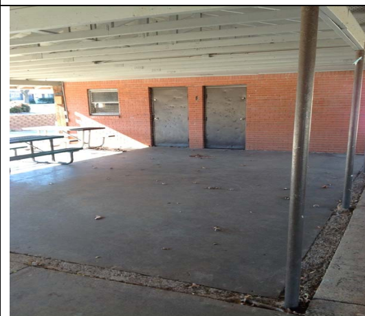
11. Comment: Violation MS_I1
