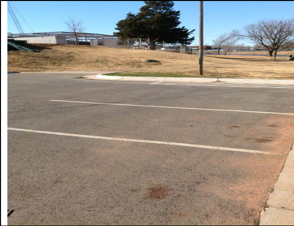
3. Comment: Violation PL_I3
