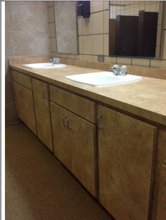
11. Even the largest restroom does not have compliant features. This lavatory does not have the required knee clearance or faucets.
