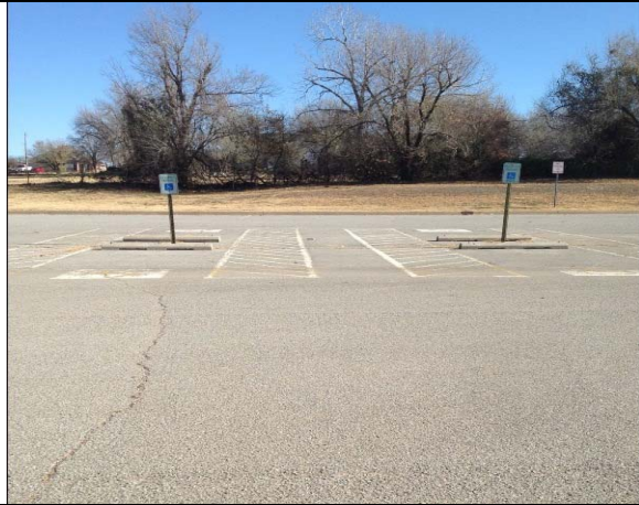
2. Comment: Violation PL_I2
