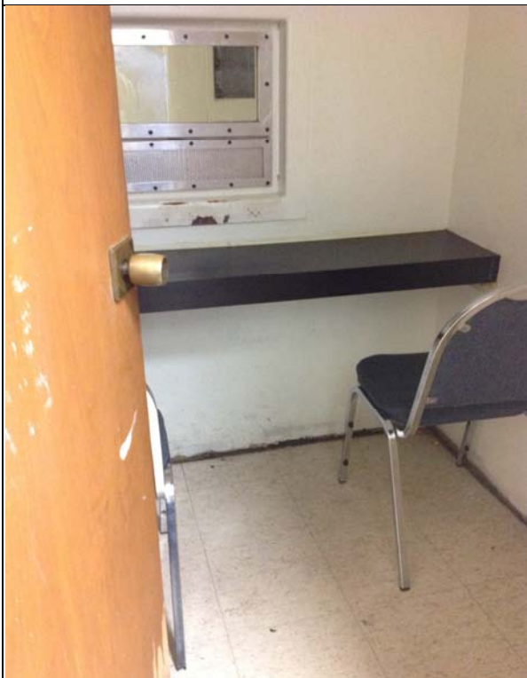
3. Cylindrical hardware needs to be replaced
