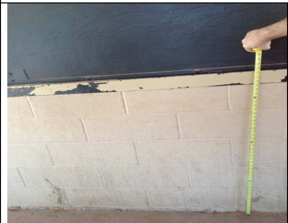
11. Comment: Violation Amn_I1
