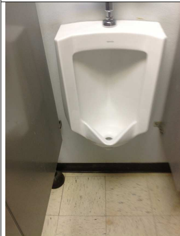
11. None of the urinals, in any of the restrooms, are compliant.
