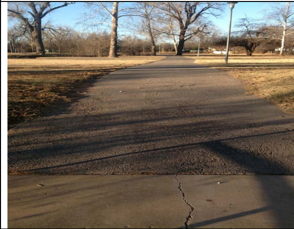
3. Comment: Violation AR_I3
