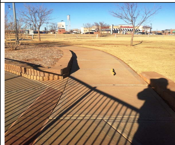
5. Comments: Violation AR_I4
