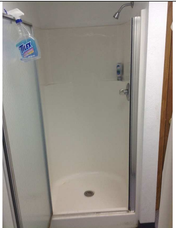
16. There are no compliant showers in the complex.
