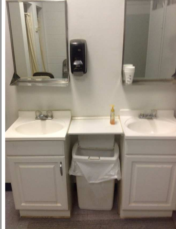
17. This restroom has no compliant features at all.
