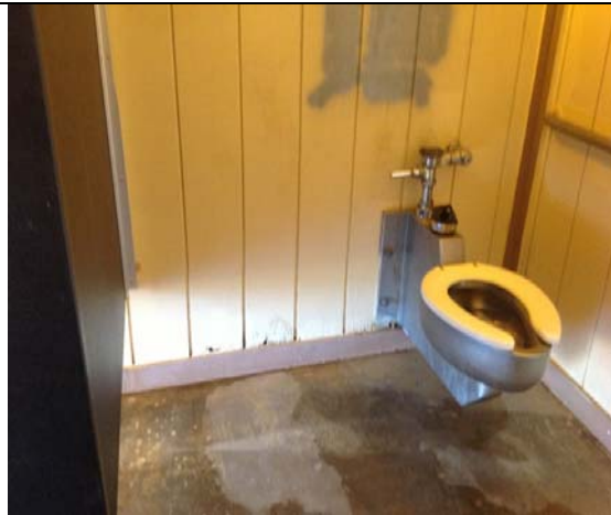
10. Comment: Violation RR_I2
