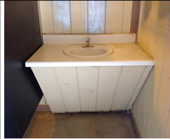
7. Comment: Violation RR_I2
