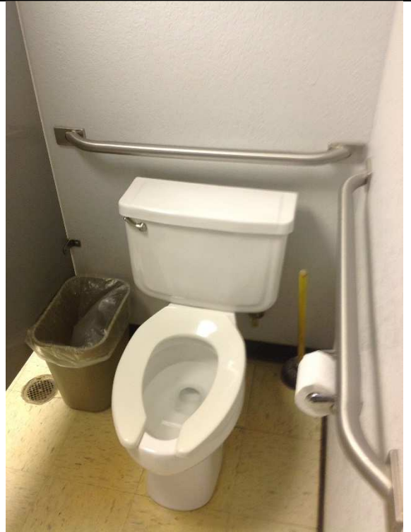
6. Although some access is attempted, the stall is not a compliant size and meets no standard.
