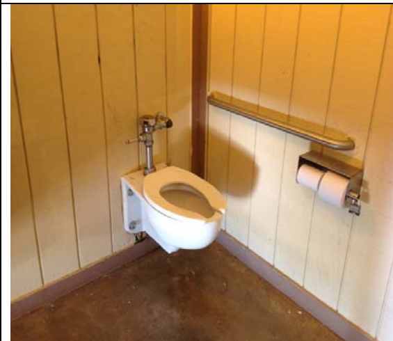
5. Comments: Violation RR_I1
