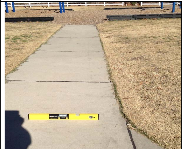
3. Comment: Violation AR_I2
