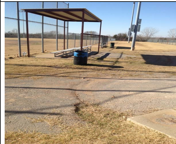
5. Comments: Violation Amn_I1
