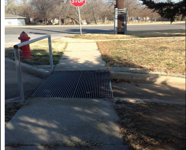
1. Comment: Violation AR_I1
