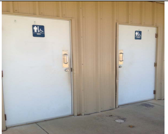
4. Comment: Violation RR_I1
