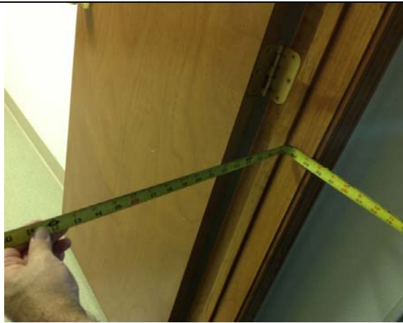
4. Comment: Violation AR_I2
