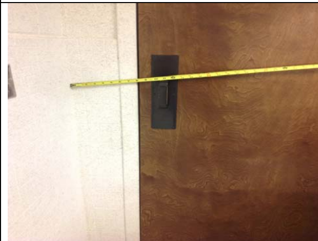
5. Comments: Violation AR_I2
