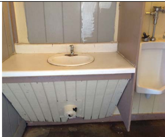
12. Comment: Violation RR_I4
