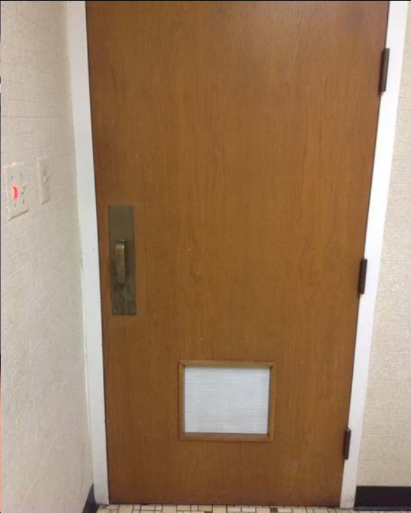
6. Restroom door maneuvering clearance.
