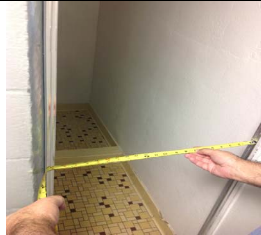
14. Comment: Violation RR_I5
