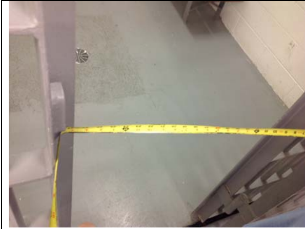
7. Comment: Violation AR_I4
