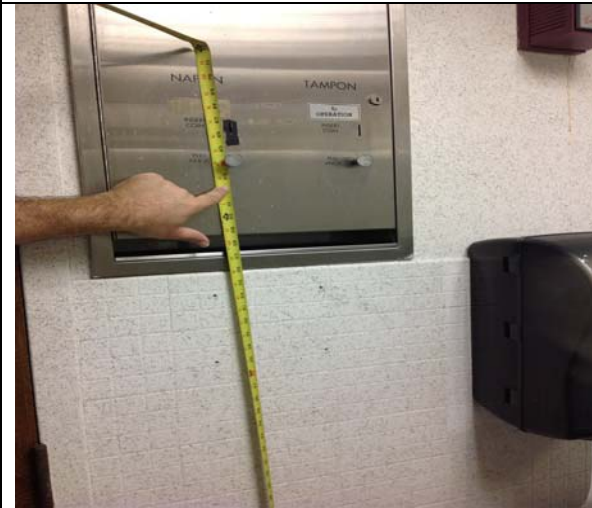
13. Comment: Violation RR_I6
