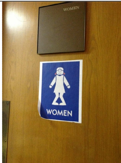
8. All signage indicating permanent spaces is required to have both raised characters and Braille. Signage will need to be replaced in this facility.
