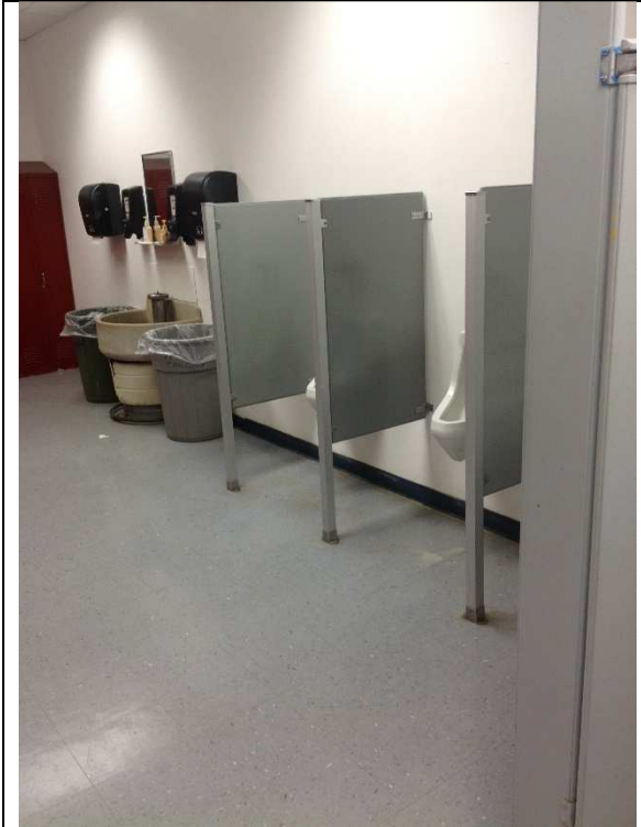
13. This men's room has no accessible features at all. A compliant urinal is 17" above the floor to the top of the rim.
