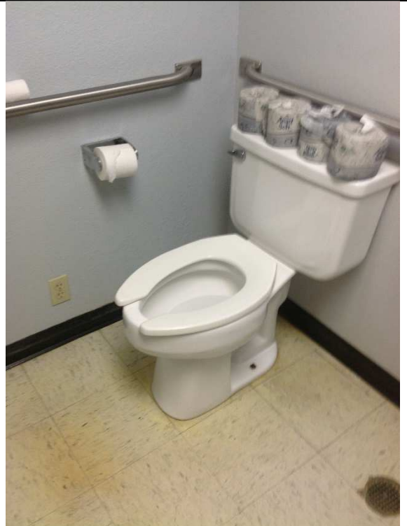
10. Even the toilet room planned for compliance has non-compliant features such as the flush control on the wrong side.
