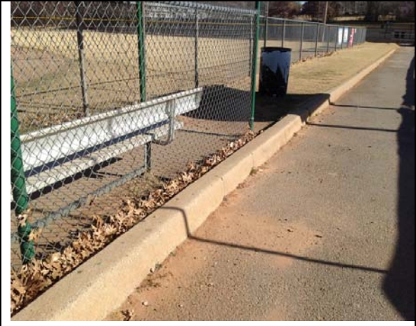
7. Comment: Violation AR_I5
