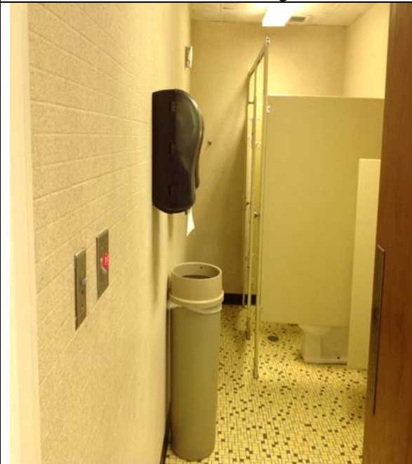
8. No accessible water closets.
