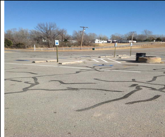
1. Comment: Violation PL_I1
