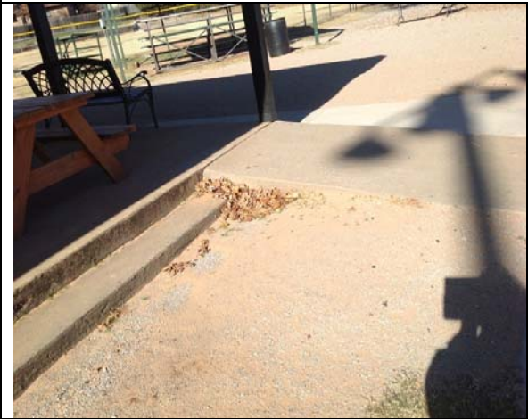
9. Comment: Violation AR_I7
