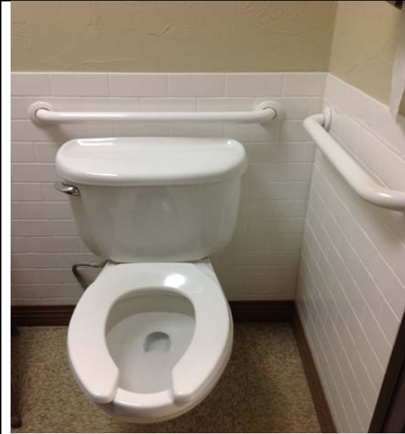
17. Single user Toilet does not have required 5' turning radius
