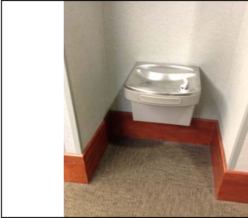
7. Comment: Violation MS_I1
