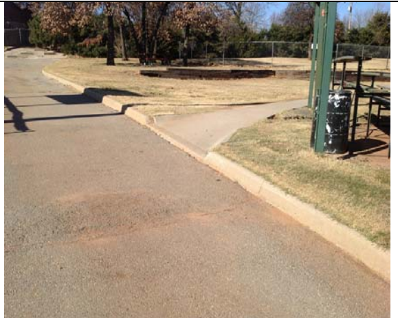
4. Comment: Violation AR_I2
