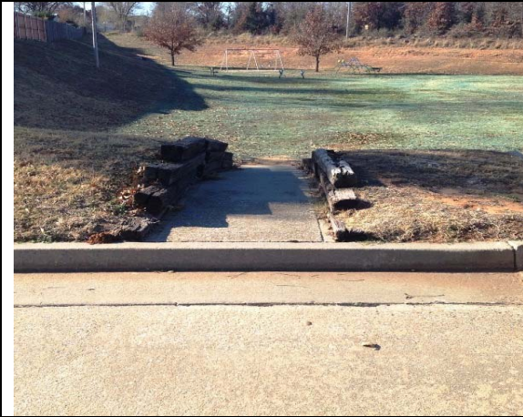
1. Comment: Violation AR_I1
