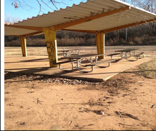
1. Comment: Violation Amn_I1
