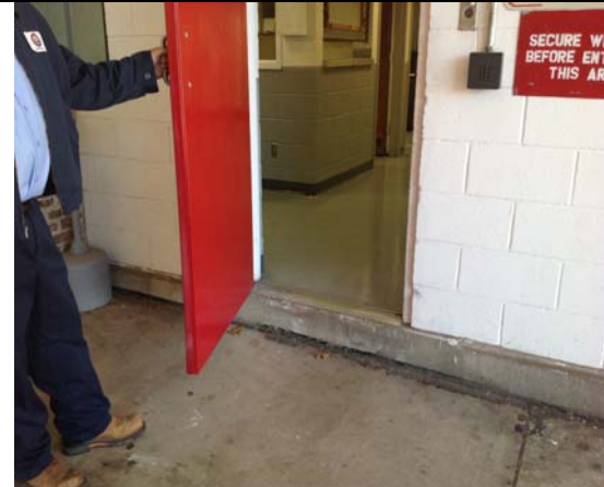
8. Comment: Violation EN_I1
