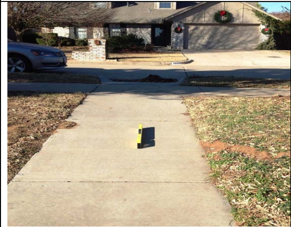
3. Comment: Violation AR_I3
