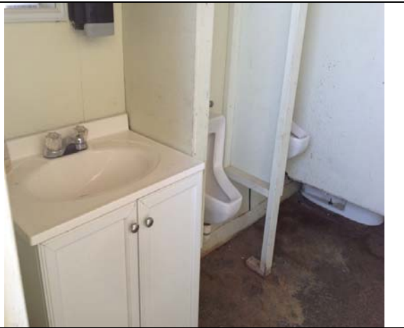
10. Comment: Violation RR_I1
