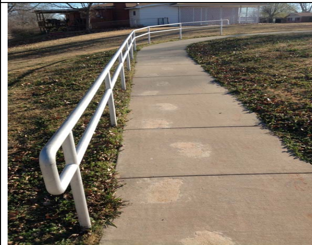
3. Comment: Violation AR_I3
