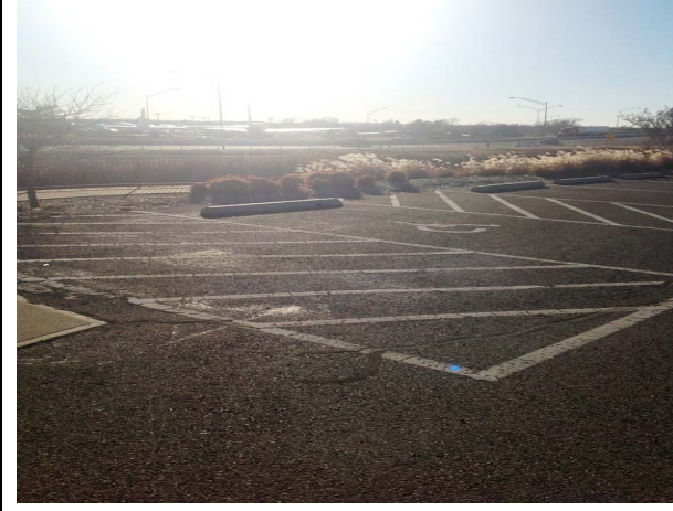
1. Comment: Violation PL_I1
