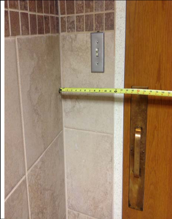
13. Door Maneuvering clearance in restroom
