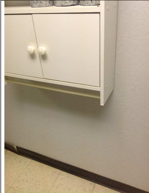
9. This is mounted in the “accessible” toilet room and is a protruding object along the path of travel.
