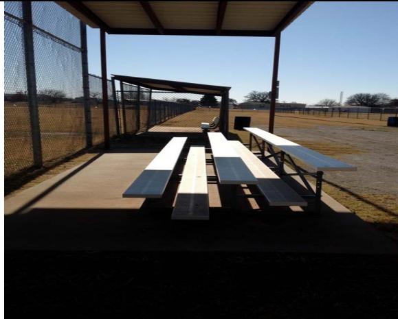
2. Comment: Violation AR_I1
