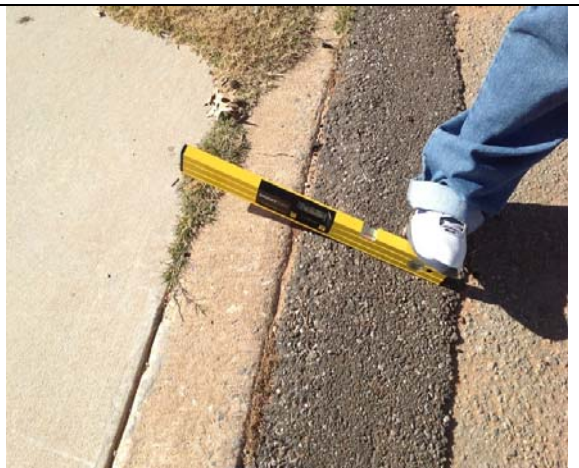
6. Comments: Violation AR_I4
