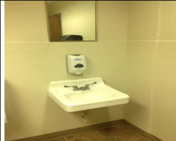
13. Comment: Violation RR_I4
