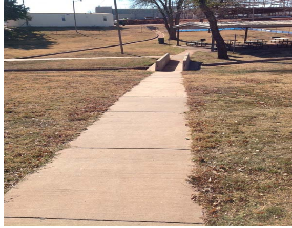
8. Comment: Violation AR_I6
