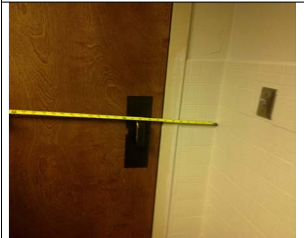
11. Comment: Violation RR_I1
