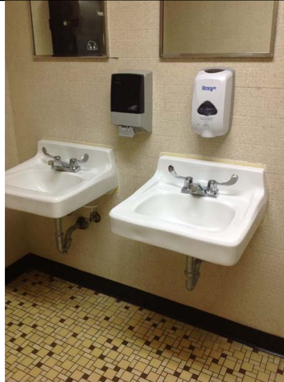
10. Water pipes are not wrapped or covered
