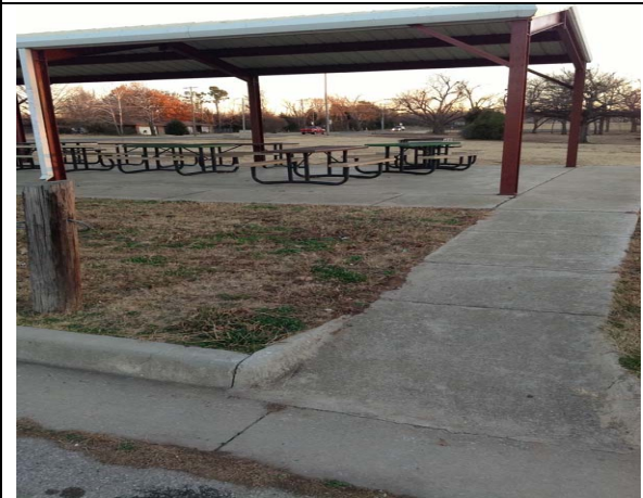
3. Comment: Violation AR_I2
