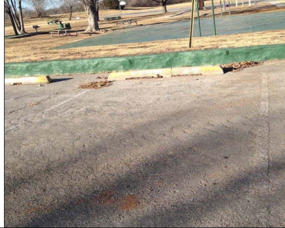
2. Comment: Violation PL_I2
