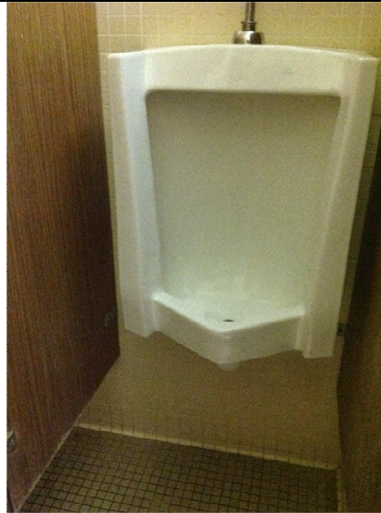
6. The urinal needs to be lowered and the path to it widened. The rim may not exceed 17" aff and the path leading to it must be a minimum of 36" wide.
