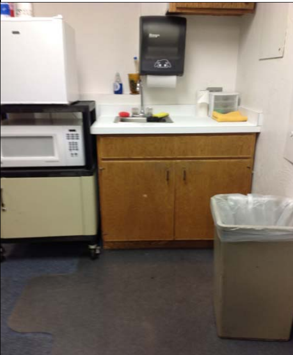
11. Break room sink has no knee clearance and counter measures at 36 in.
