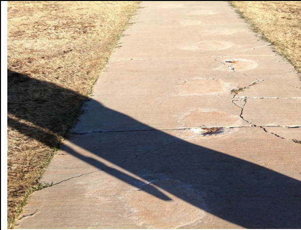
1. Comment: Violation AR_I1
