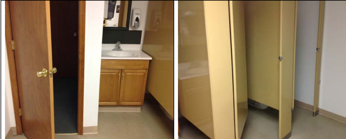
7. Comment: Violation RR_I2
