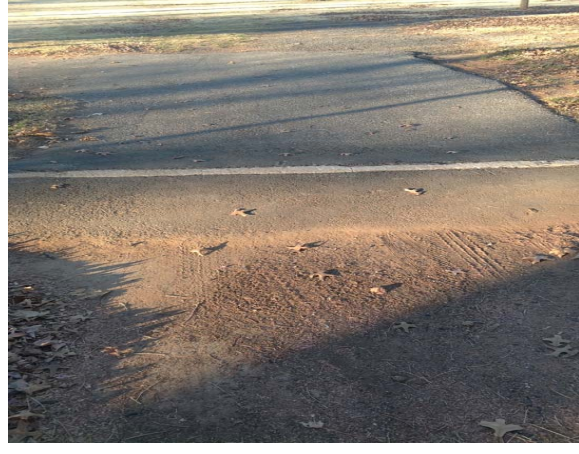
2. Comment: Violation AR_I2
