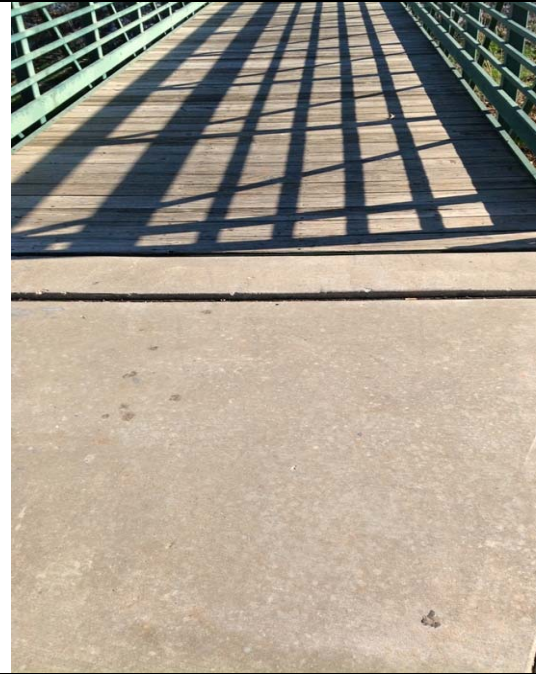
2. Comment: Violation AR_I2
