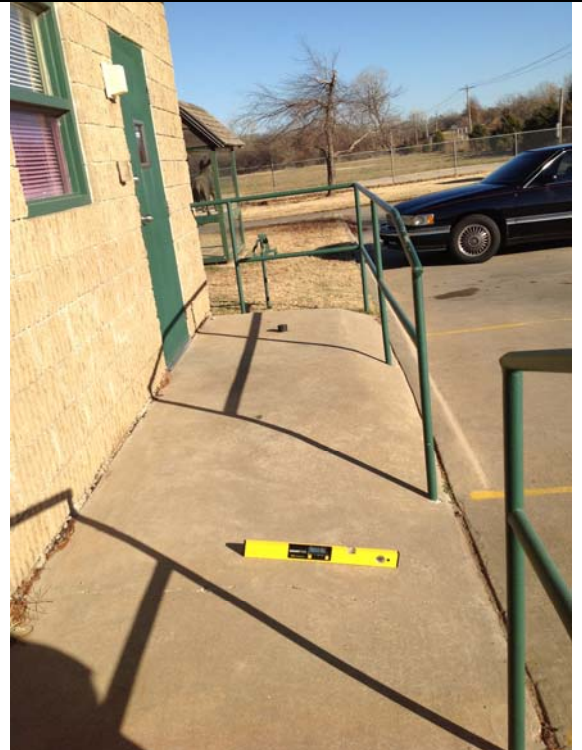
2. Severe slope to entry
