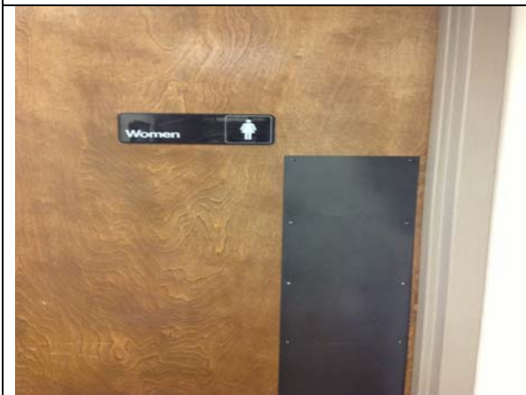
9. Comment: Violation HW_I1
