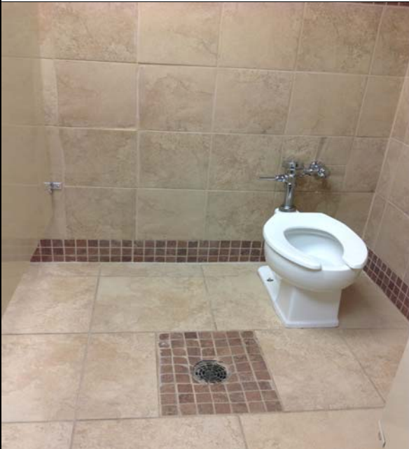
15. Water closets not compliant
