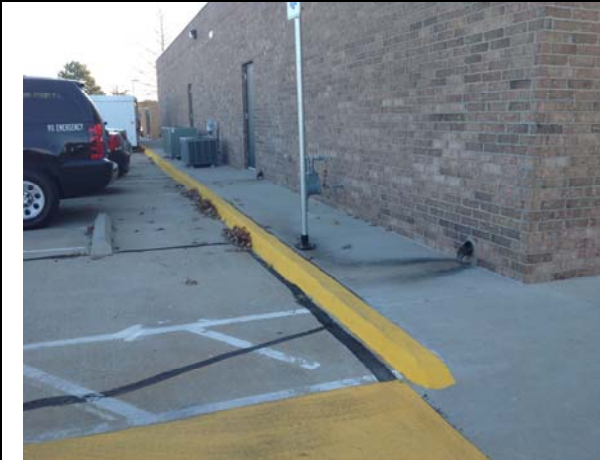
1. Comment: Violation PL_I1
