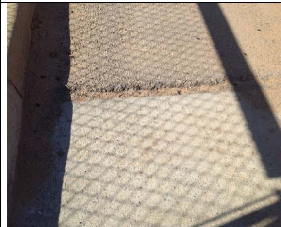
5. Comments: Violation AR_I3
