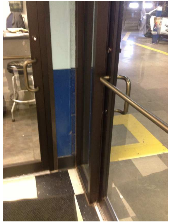
2. Doors in main work areas also do not have the required maneuvering clearances.
