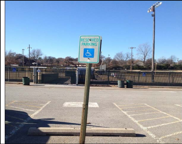
1. Comment: Violation PL_I1
