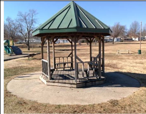
3. Comment: Violation AR_I3
