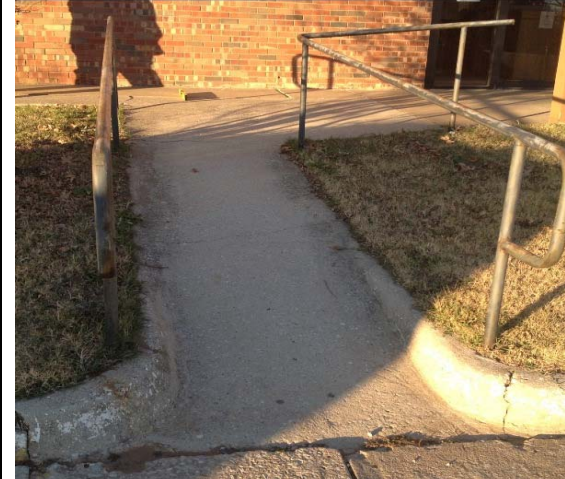
1. Comment: Violation PL_I1
