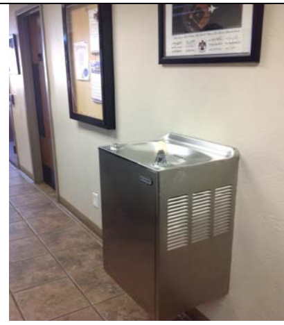
14. Comment: Violation MS_I2
