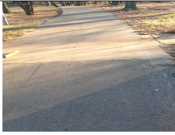
6. Comments: Violation AR_I6
